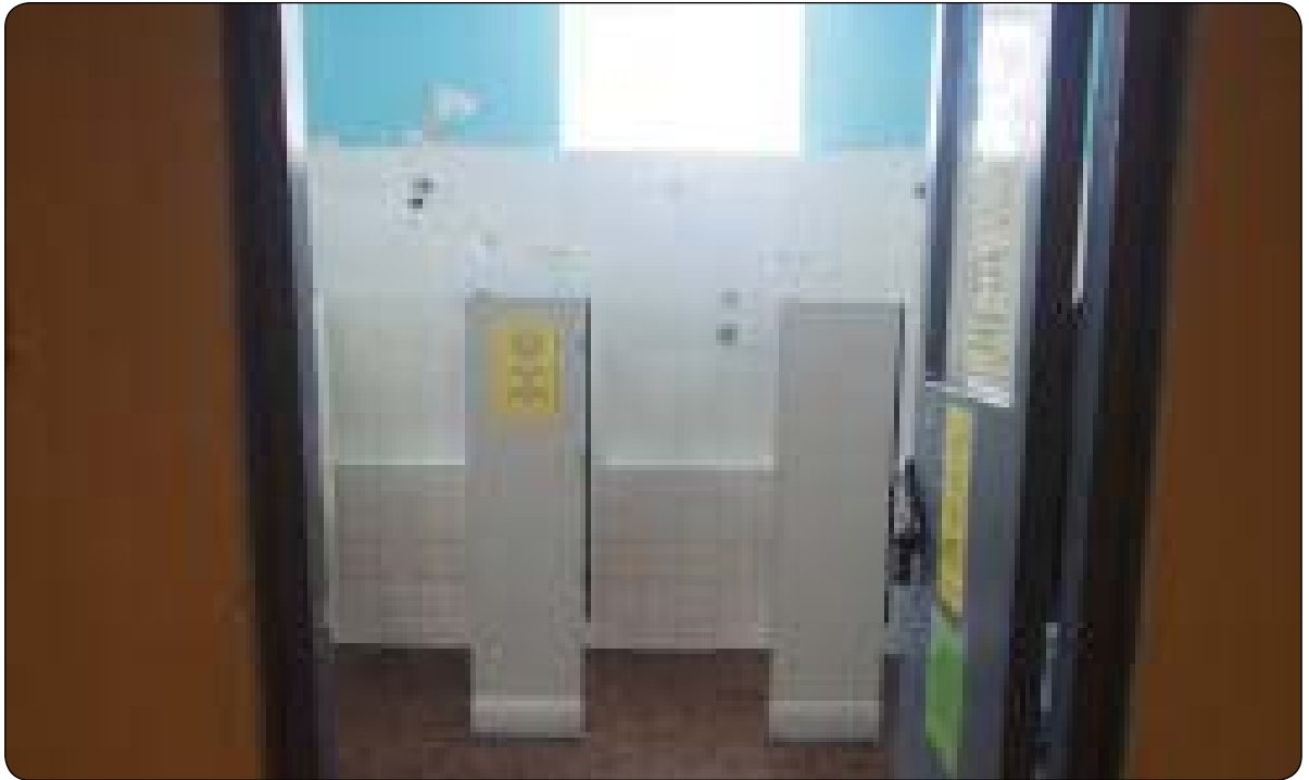
Communal shower blocks at MSPC 3 with trip hazards and slippery surfaces.
