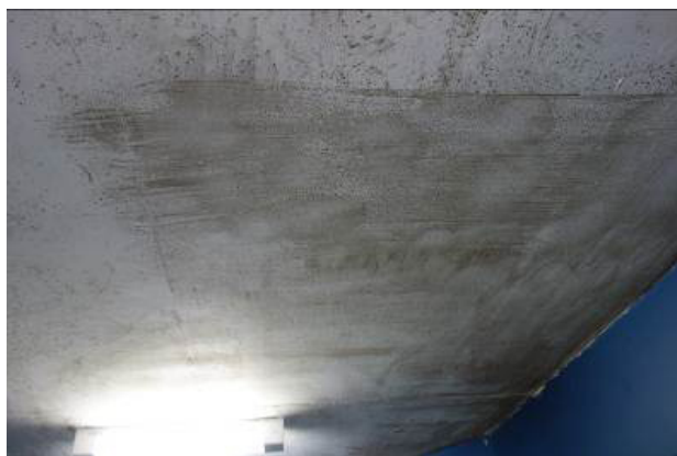
Mould on ceiling in cell
