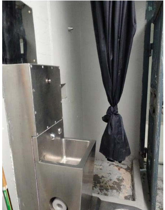
Segregation cell shower and sink
