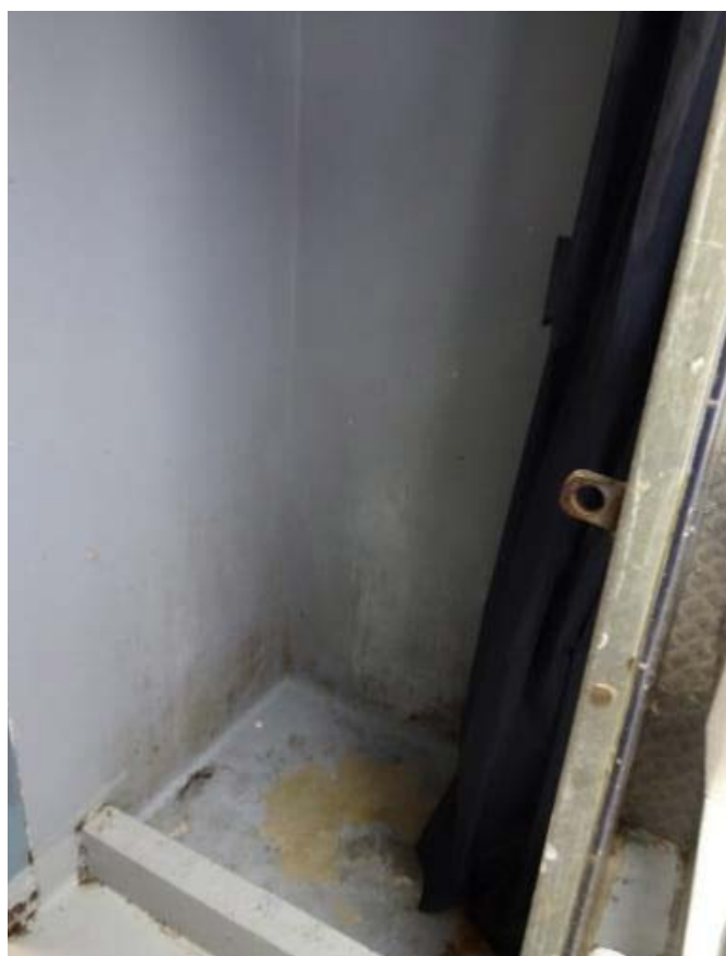
Shower in cell, induction unit
