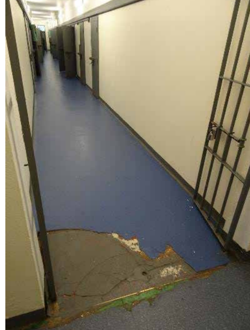
Damaged flooring in the minimum security accommodation
